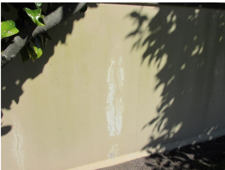
Stucco perimeter wall paint finish deterioration
