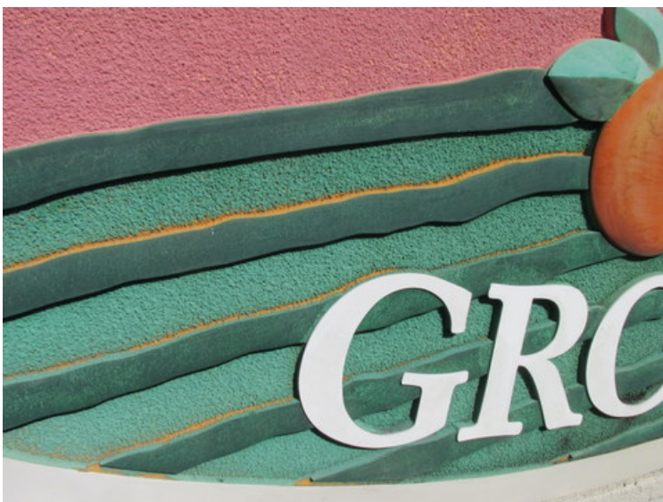
Entrance monument paint finish deterioration
