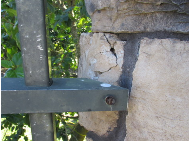
Aluminum fence fastener displacement and masonry deterioration noted at entrance monument
