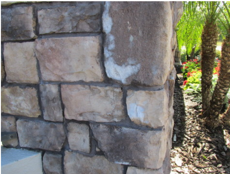
Masonry efflorescence noted at entrance monument
