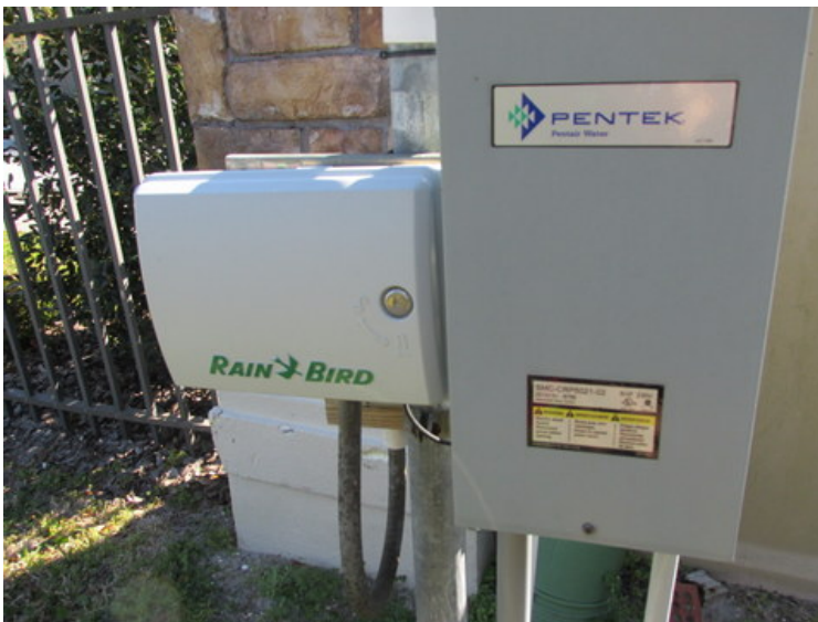
Irrigation system controller
