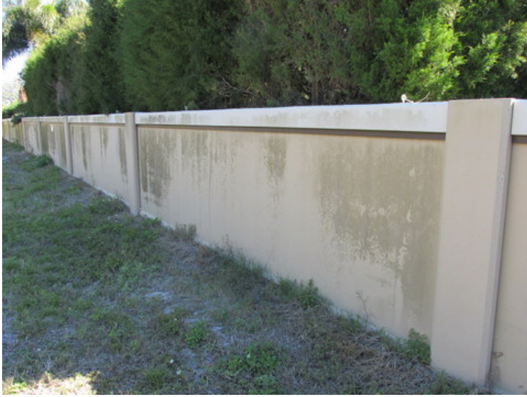
Stucco perimeter wall stains and paint finish deterioration
