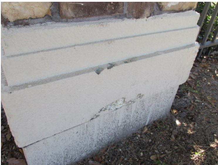
Stucco deterioration noted at base of masonry columns
