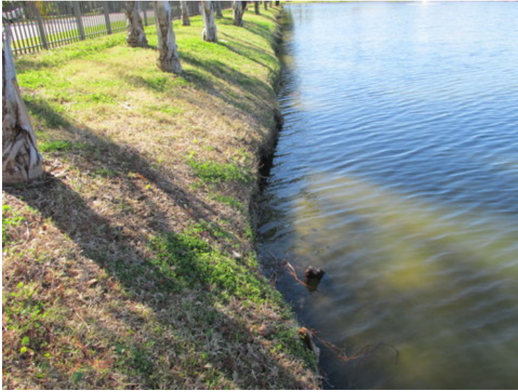
Minor pond shoreline erosion
