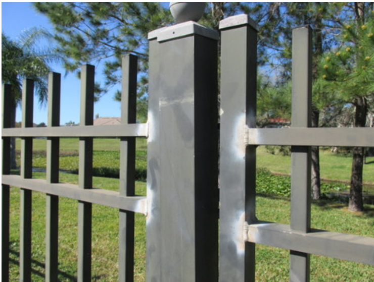
Aluminum fence finish deterioration
