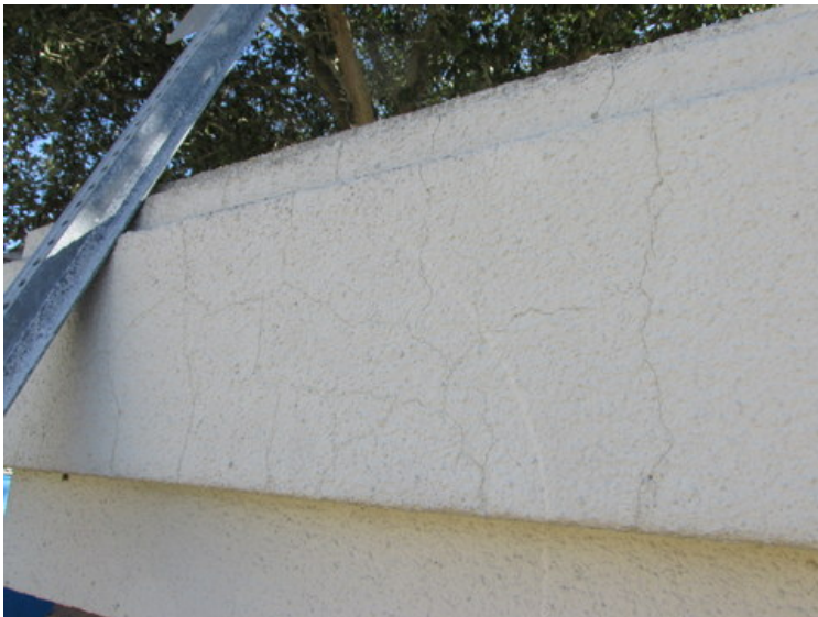
Stucco perimeter wall cracks
