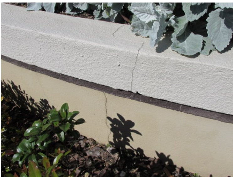
Stucco cracks noted at entrance monuments
