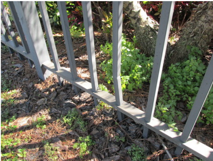
Minor aluminum fence damage
