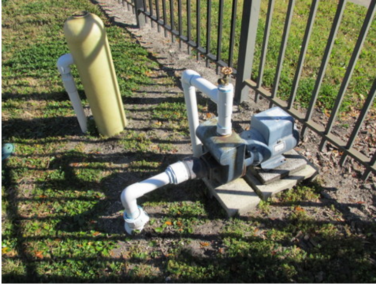
Irrigation system pump
